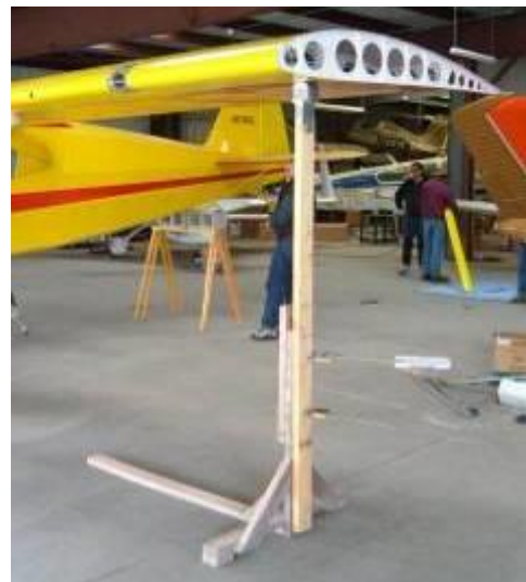
With the left wing bolts in place, a 2x4 was clamped to the rotisserie stand to hold up the wing while the other wing was being installed. Something about lateral asymmetry out of limits. The top of the 2x4 was padded with foam liberated from the packing boxes of new computers at TPS.
